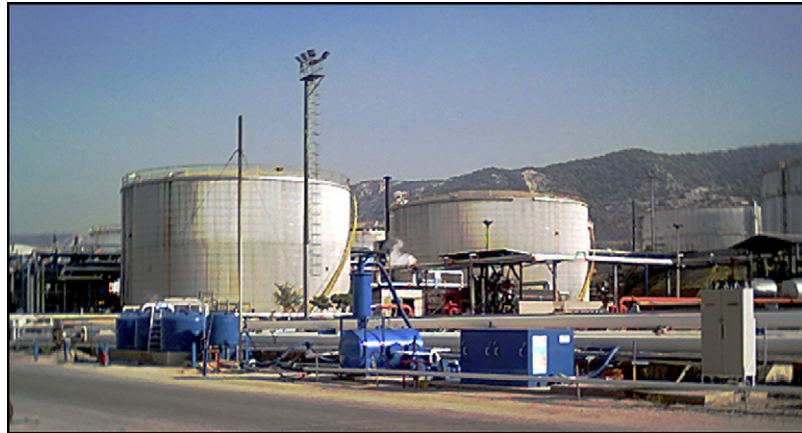
Fig. 4. View of the installed bioslurping system.
